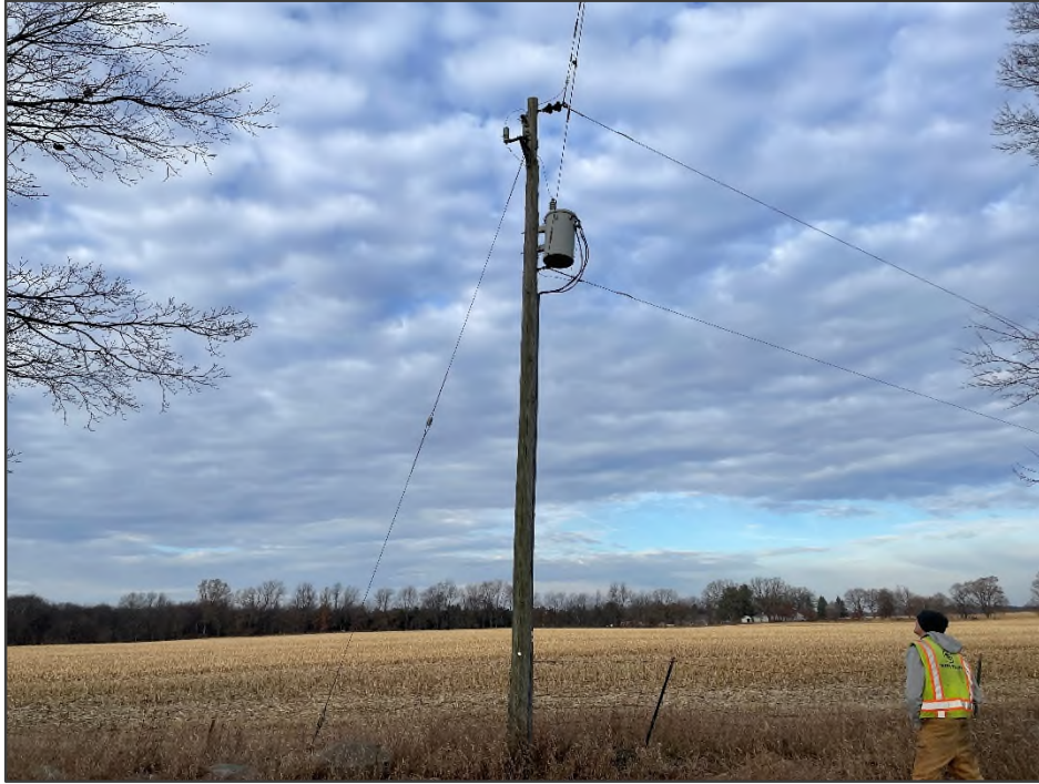
PHOTO NO. 11: View of a typical pole-mounted transformer.
