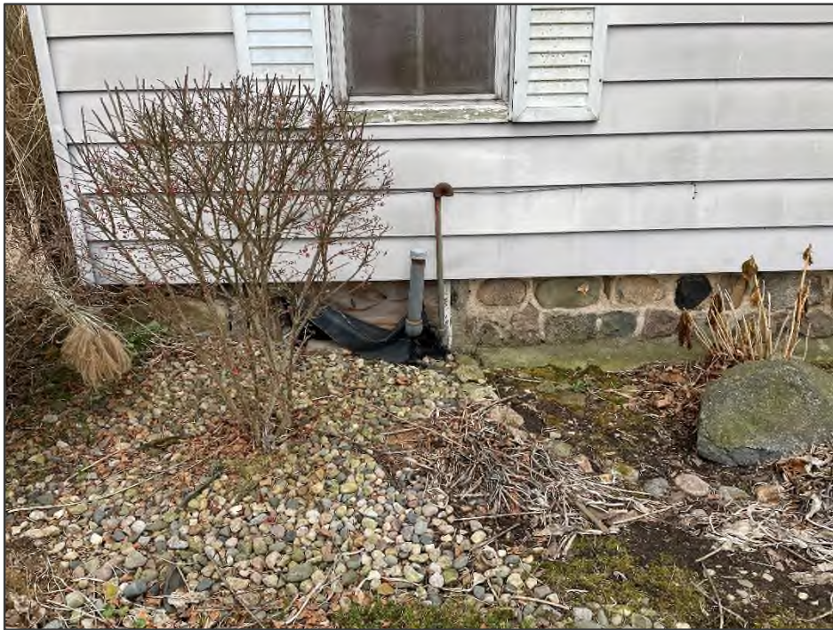
PHOTO NO. 30: View of the potential heating oil tank vent and fill pipes extending into the basement of the residential structure at 16-282-003-00 (14716 C Drive North).
