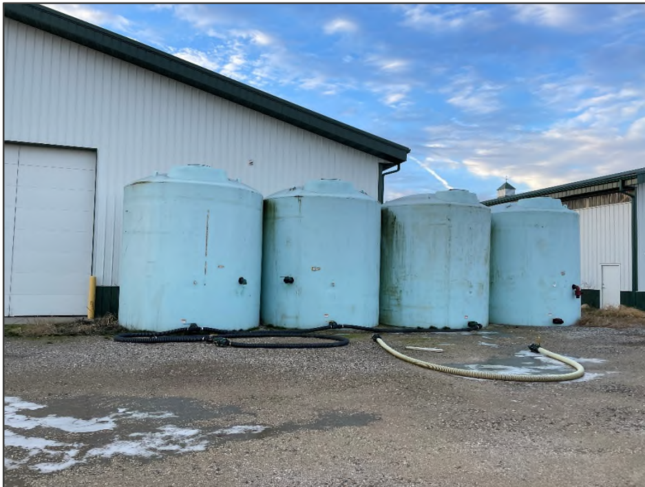
PHOTO NO. 14: View of the four, 10,000-gallon pesticide and water tanks located north of the structure at 16-281-021-00 (14219 C Drive North).
