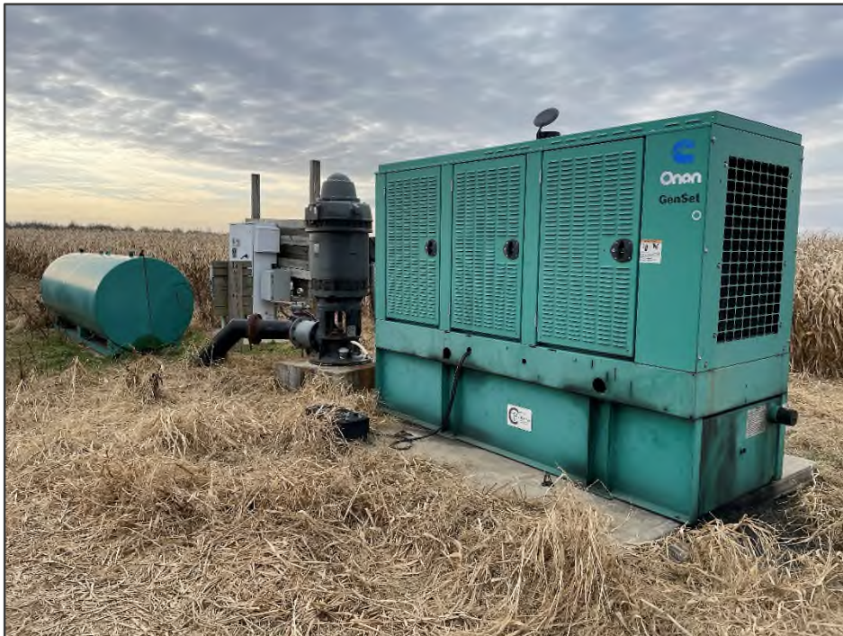
PHOTO NO. 18: View of the generator, groundwater well, and 3,000-gallon fuel AST located near the center of 16-291-009-00.
