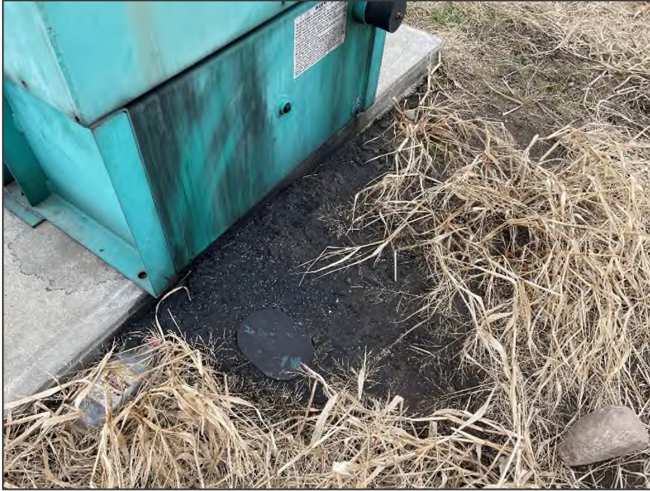
PHOTO NO. 19: View of the stained soil near the generator.
