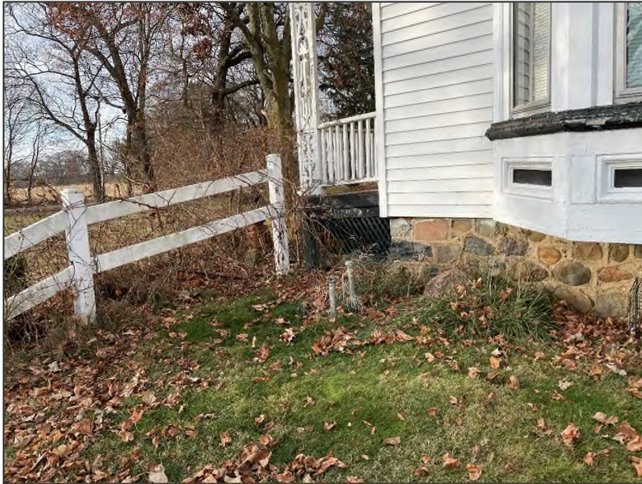
PHOTO NO. 23: View of the potential heating oil UST vent and fill pipes located at 16-290-018-00 (13315 C Drive North).
