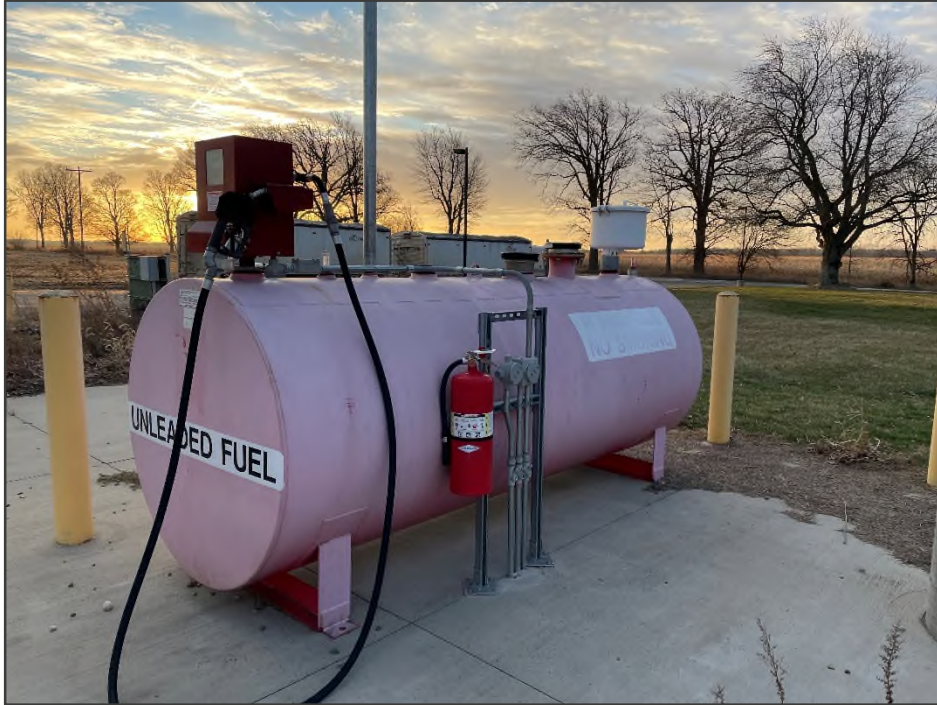
PHOTO NO. 13: View of a 3,000-gallon fuel AST located south of the structure at 16-281-021-00 (14219 C Drive North).
