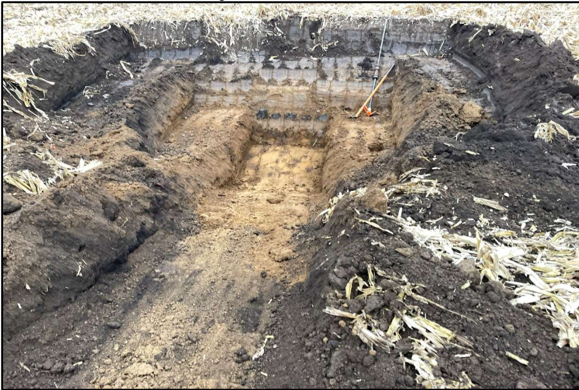
PHOTO NO. 2: Test Pit TP319 facing north. Re-excavated later to improve 7' by 7' area.
