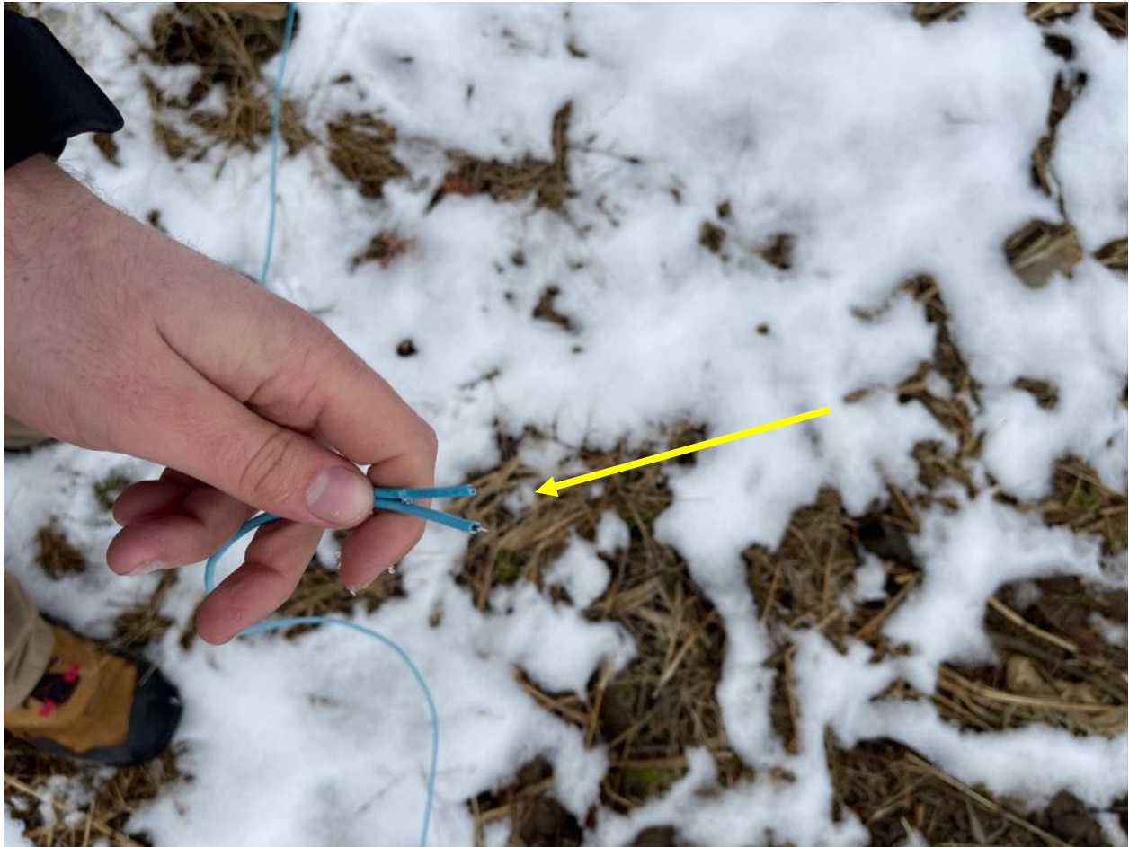
Figure 8. Cabling damaged on site (yellow arrow).
